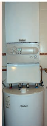
Boiler & Cylinder by Andy Butler is licensed under CC BY 2.0
